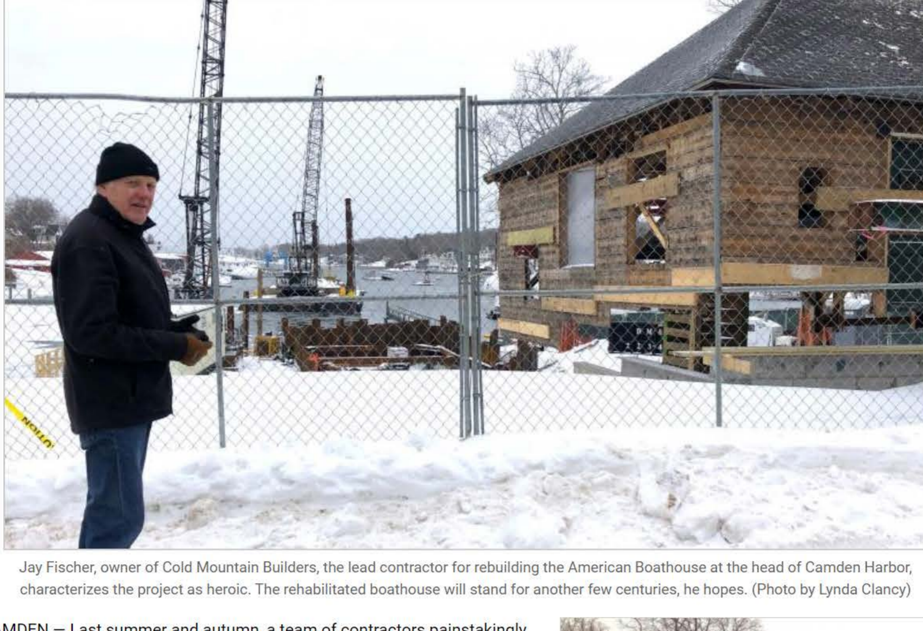
Jay Fischer, owner of Cold Mountain Builders, the lead contractor for rebuilding the American Boathouse at the head of Camden Harbor, characterizes the project as heroic. The rehabilitated boathouse will stand for another few centuries, he hopes. (Photo by Lynda Clancy)
